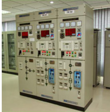
Figure 5.3: Control, metering & relay panels [6].
