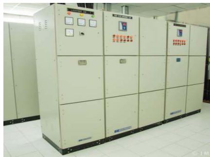
Figure 5.4: Power Factor Improvement (PFI) Plant [6].
