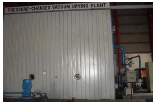
Figure 4.10: Vacuum Drying Plant
